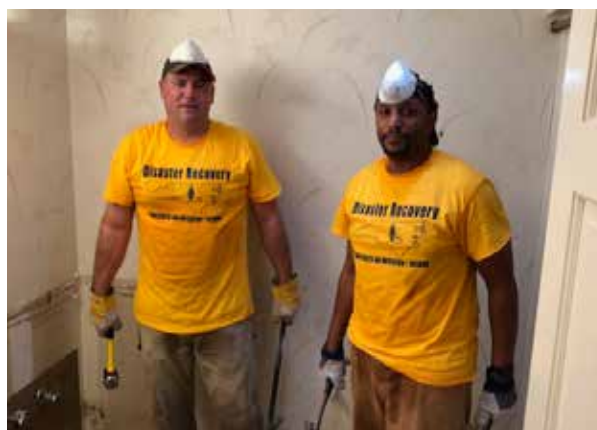
AgCarolina employees Roy Robertson and Antoine Moore gutting a house in the New Bern area.
